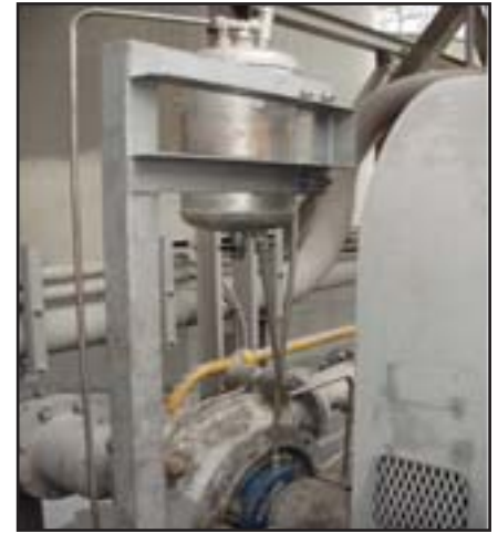
AESSEAL® water management system on slurry pump duty.
